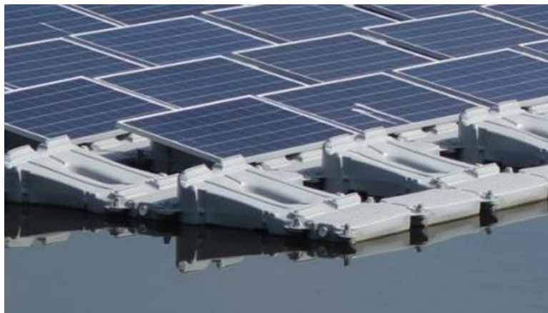
Fig. 11 - a flotovoltaic panel demonstration project
